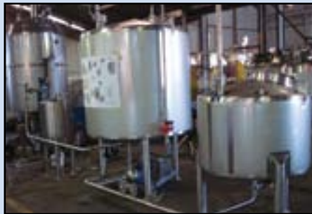
CIP system pipework - factory set up
