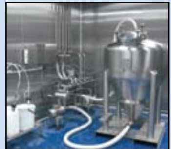
750 ℓ Portable storage vessel in wash bay
