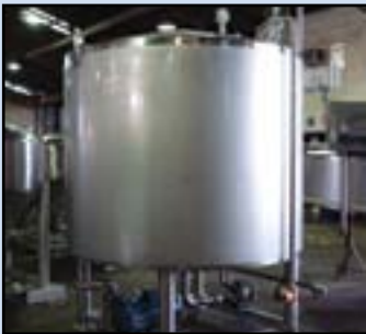
3000 ℓ Hot water tank with vacuum pump
